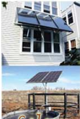
Solar PV Systems
